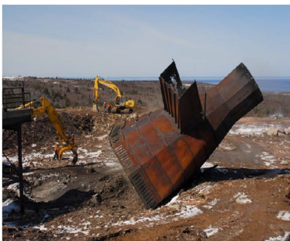
Incinerator in Old Perlican being dismantled and replaced with a waste recovery facility
